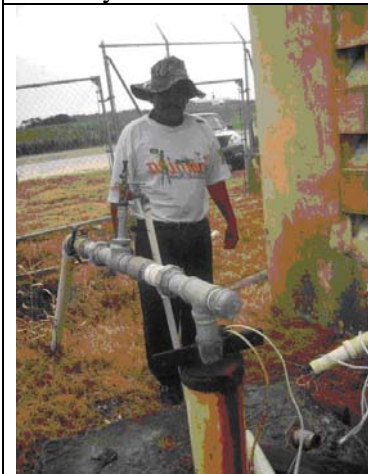
Well and line to water tank
