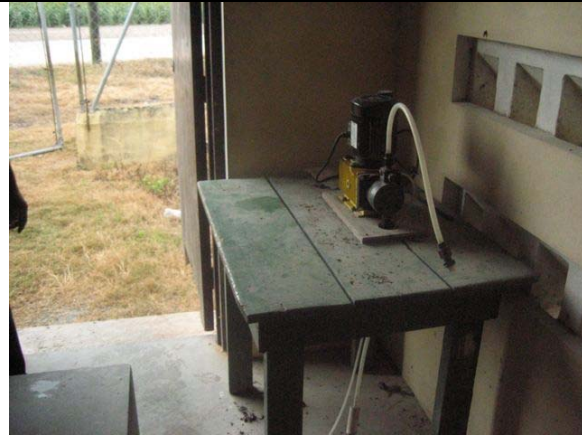
Chlorine injection pump (not currently used)
