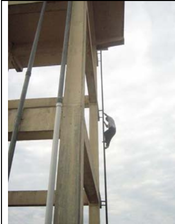
Roberto Coye, Water Board, checking water level in tank
