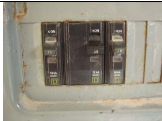
Breakers for pump and lights
