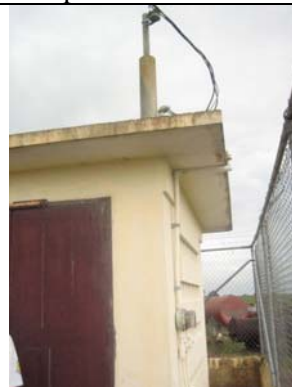
Service entry at pump house
