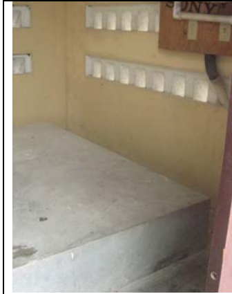
Concrete base in pump house, electrical gear on wall
