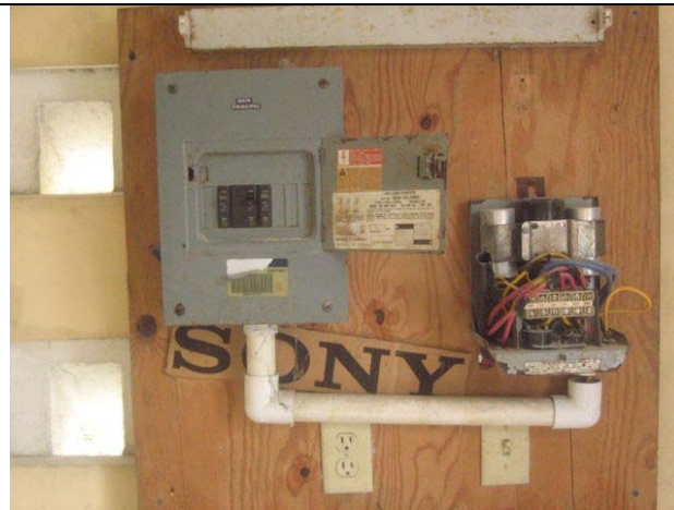
Electrical panel and pump control
